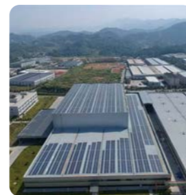
Guojing Pharmaceutical PV Power Station
